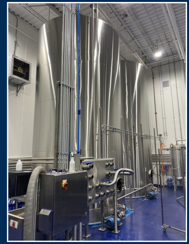
2 Stainless steel tanks Cap.: 44 500 L each
