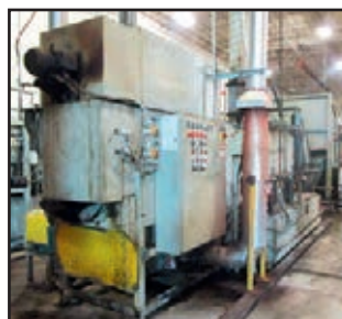
2002 ALMCO/PINTURA FINISHING 30-WRD-G PARTS WASHER/DRYER
