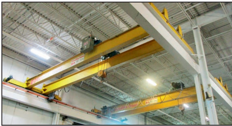
(2) CANADIAN CRANES 10-TON X 36' (EST) OVERHEAD BRIDGE CRANES
