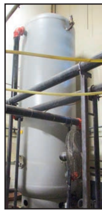
(1 OF 2) AIR RECEIVER TANKS
